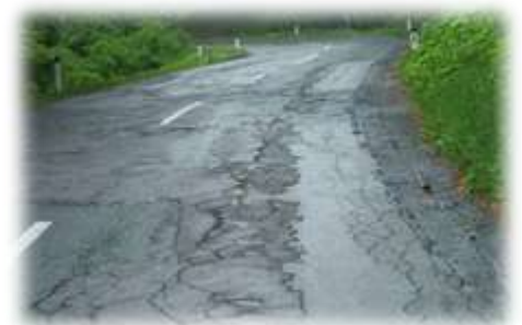
Figure 2.3 Deteriorated low volume road
